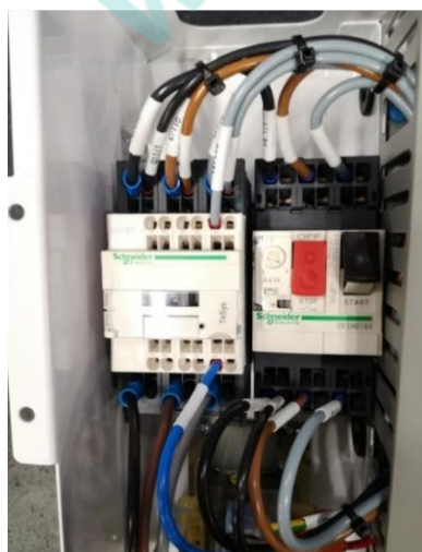
Figure 18: Main switch & overload protection C6.1.10/0618-1019/E
