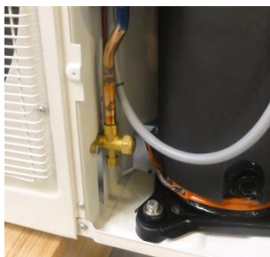
Figure 23: Liquid line service port
